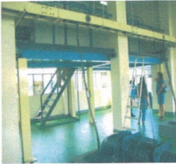
Figure 5 Elevated Controller at BPS Macasandig
