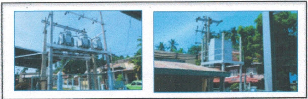
Figure 7 Elevated Transformers at BPS Macasandig
